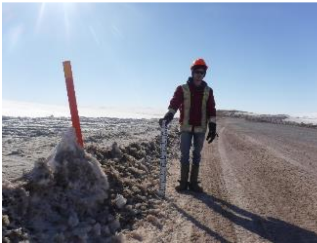
Photo 13 Example of snow bank management on east and west sides of Tote Rd to ensure they do not exceed the maximum snow depth, May 13, 2018.
