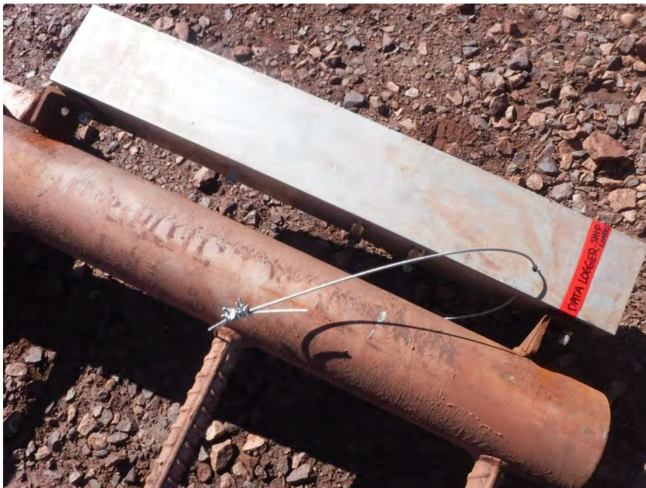
Figure 5: Hardware attaching aluminium tube to steel L brackets and wire rope for redundancy of the L bracket attachments.
