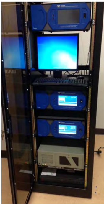
Photo 1-6 The rack-mounted Teledyne T100 (SO 2 ) and T200 (NO x -NO 2 ) continuous gas analyzers at the PSC
