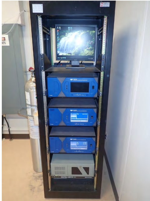
Photo 1-2 The rack-mounted Teledyne T100 (SO 2 ) and T200 (NO x -NO 2 ) continuous gas analyzers at the MSC
