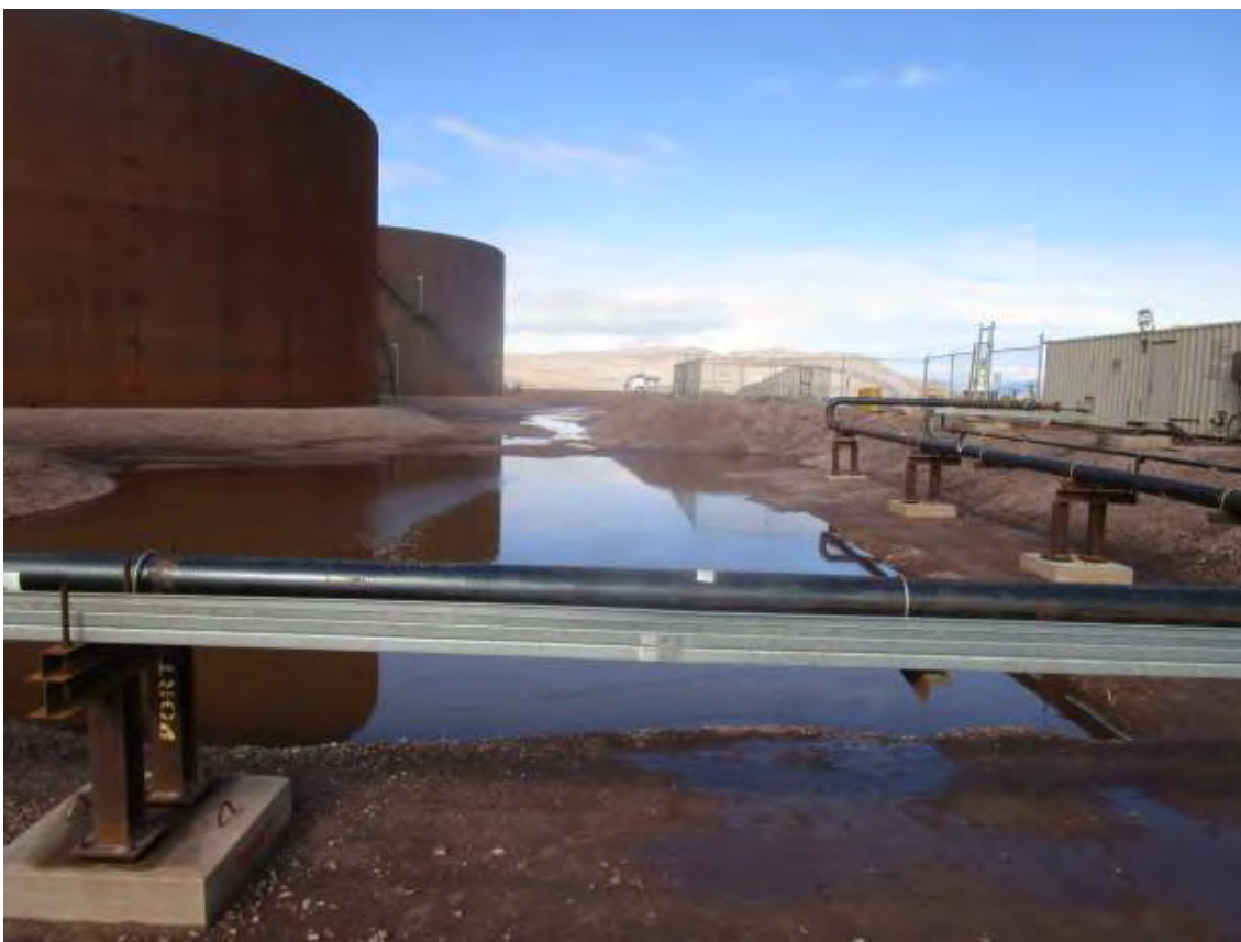
2. Port Site Fuel Tank Farm
