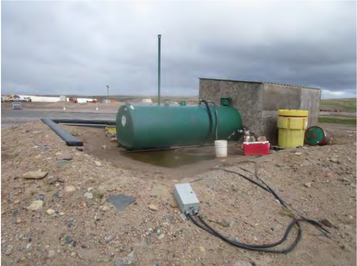
6. Helicopter Fuel Cell Containment
