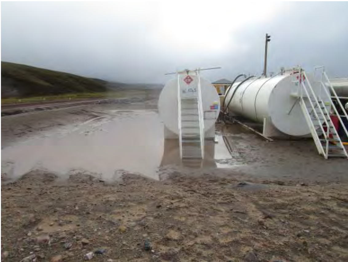
11. Jet Fuel Pump and Tank Containment
