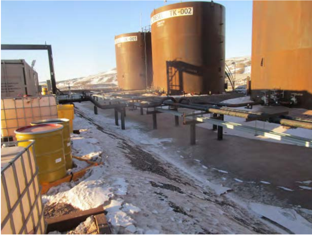
M. Mine Site Fuel Tank Farm Containment
