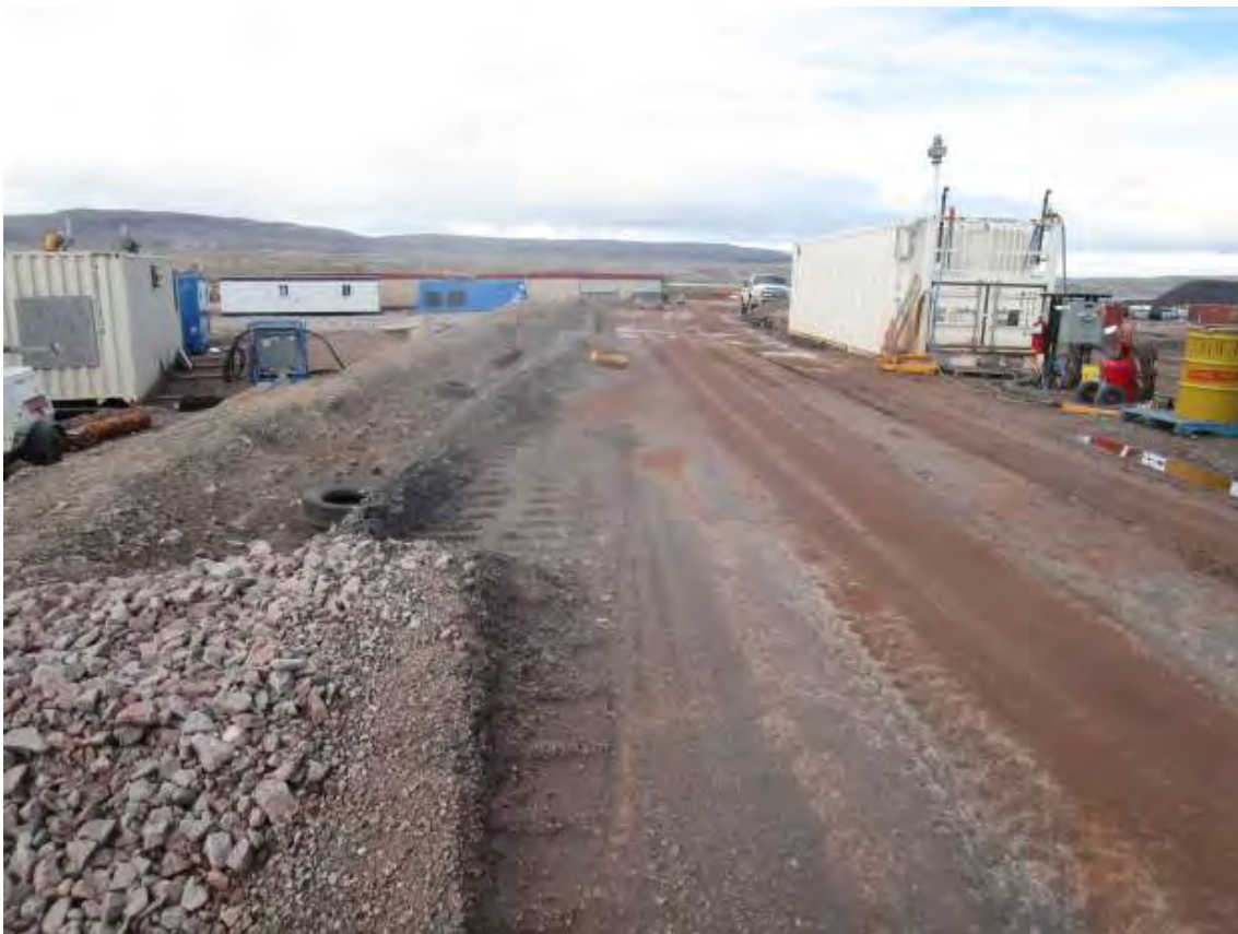
10. Fueling Facility Containment
