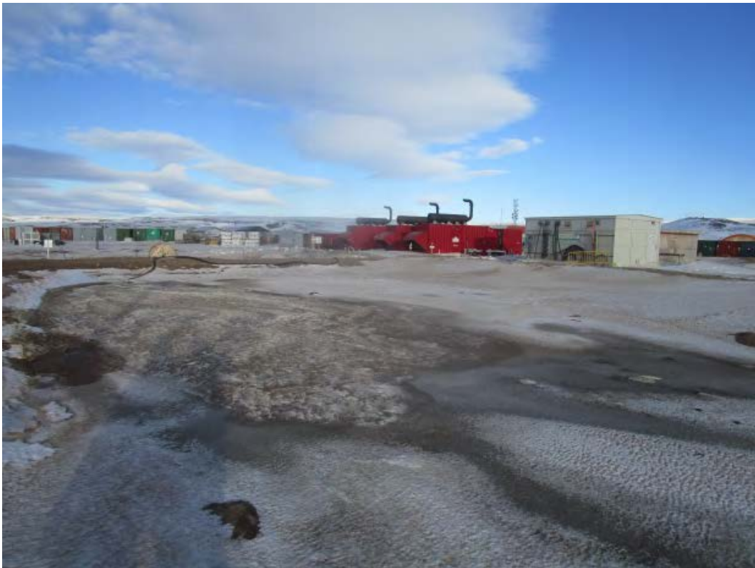
B. Generator Fuel Storage Containment
