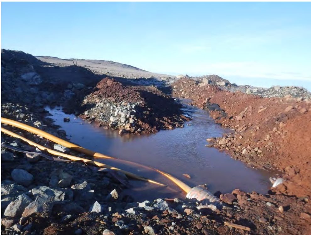
Photo 2. June 20 th , 2018 – West drainage ditch inflow into the Waste Rock Stockpile Pond following berm reinforcement.
