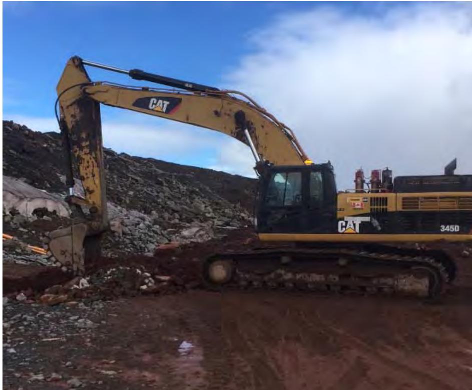
Photo 1. June 19 th , 2018 -Heavy equipment support upon discovery to arrest over flow from West Drainage Ditch.
