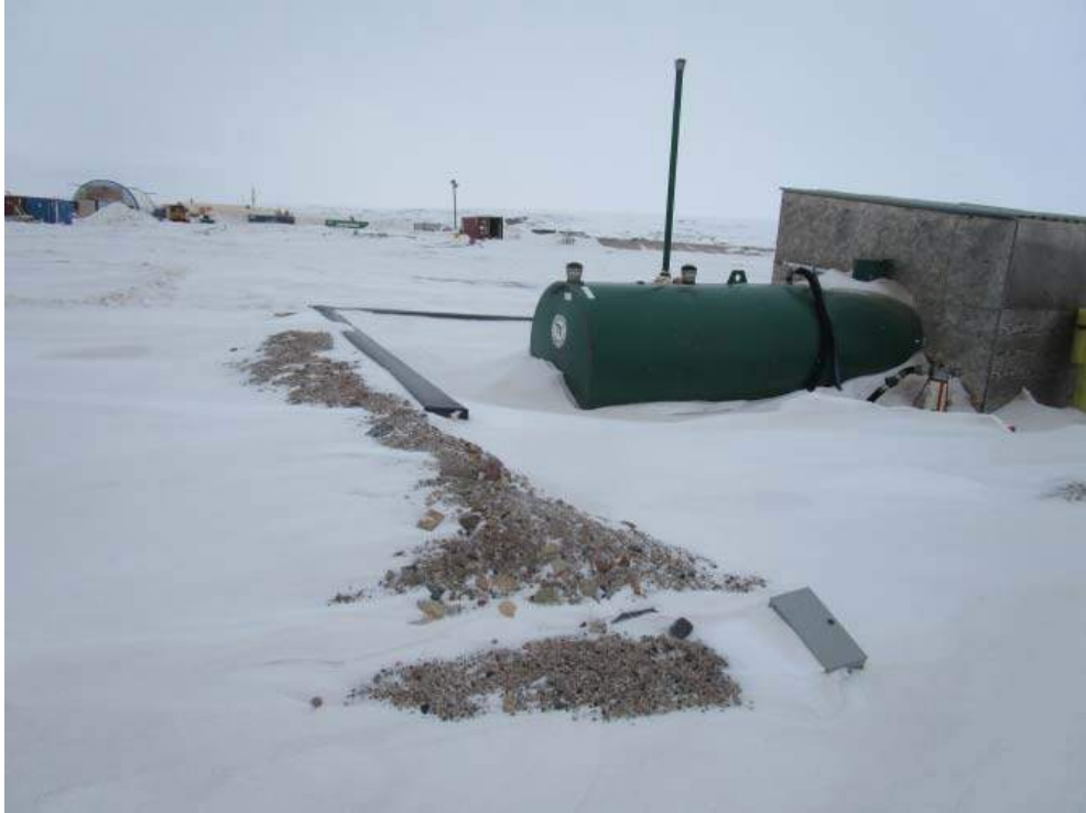
Helicopter Fuel Tank Containment
