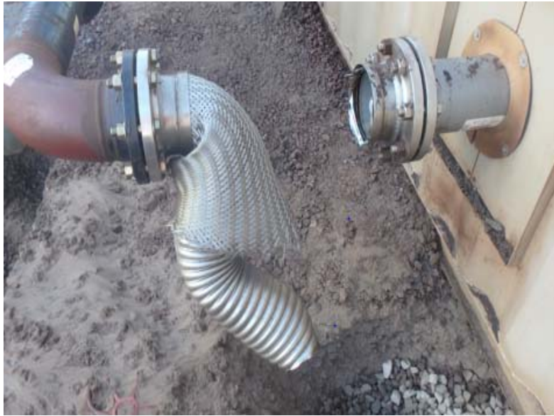
Photograph 1 – Braided Flex Pipe fuel supply line to back of Module
