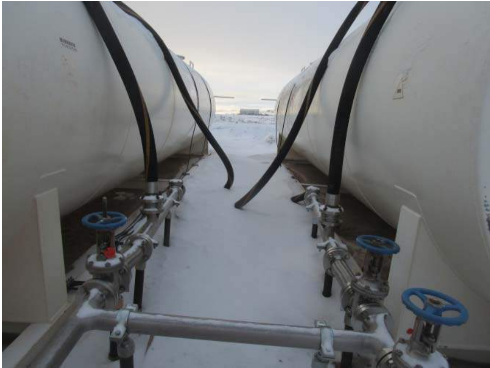
Jet "A" Fuel Containment
