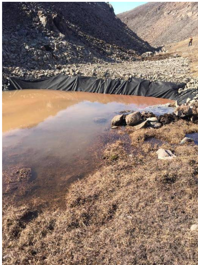
Photo 6 – Check dam constructed at outlet of Sheardown Valley along Mine Haul Road.
