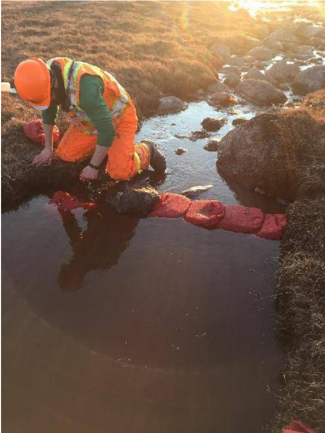
Photo 4 – Sand bag check dams installed along Sheardown Lake Tributary LDFG near landfill access road.
