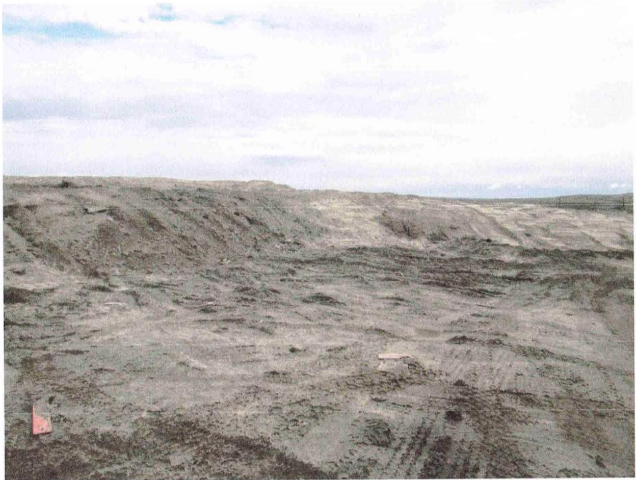
Solid Waste Disposal Site. Dyke to contain waste on edge of second lift.
