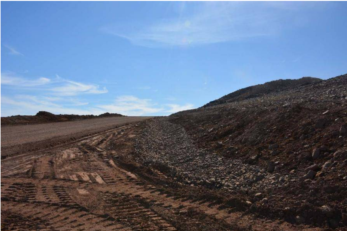
Photo 4 - New ditch with geotextile and rip rap at downhill from Km 108.5. Picture taken on July 5, 2016
