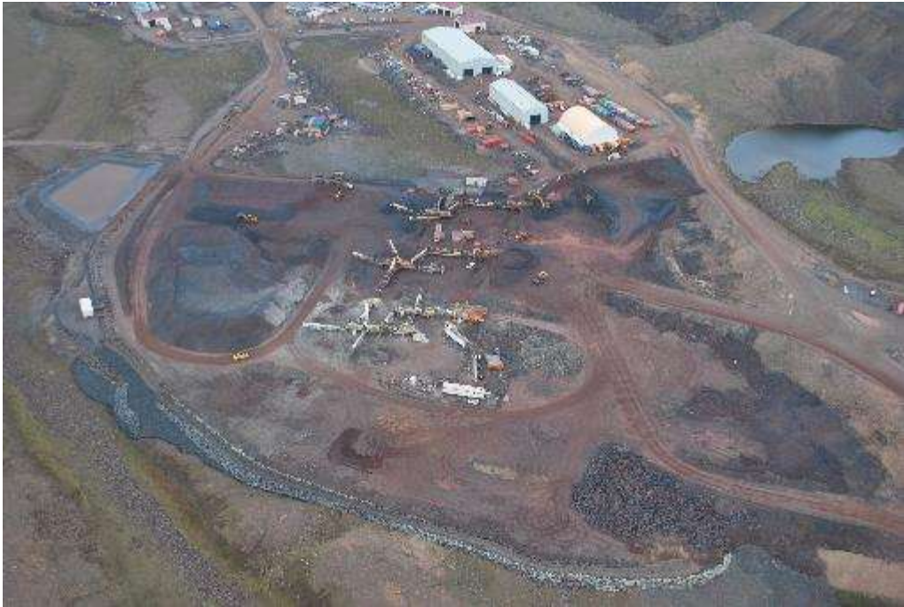
Photo 1 – Aerial view of completed ditch work at the Mine Site Crusher Pad on July 18, 2016
