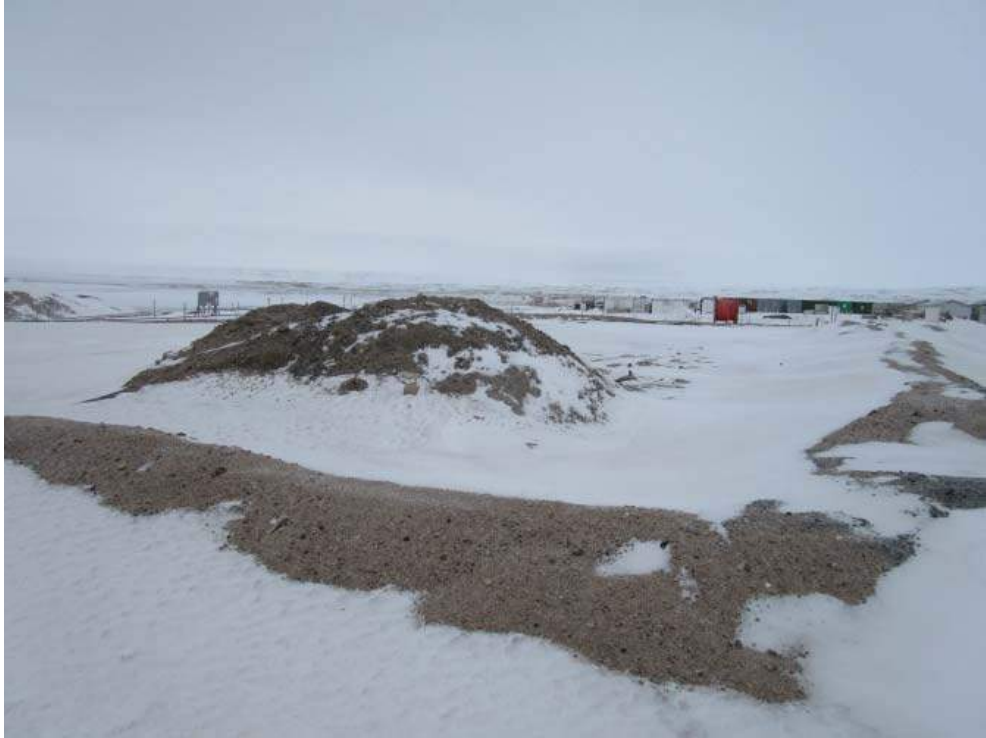
Generator Fuel Storage Containment
