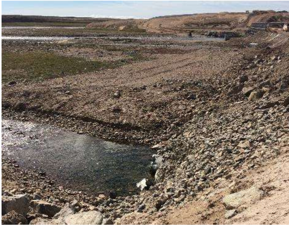
Photo 1 – Water flowing downstream of CV223 on July 22, 2016
