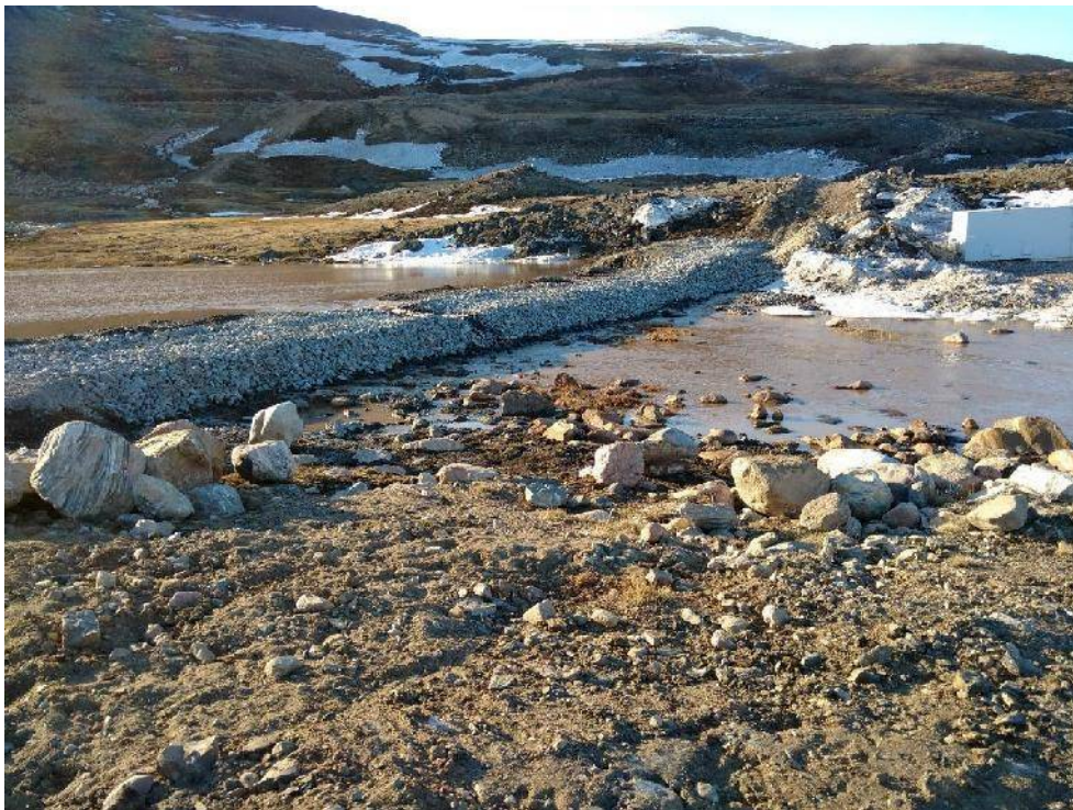
Photo 2 – Mine Haul Road runoff pooling upstream of Check Dam # 4
