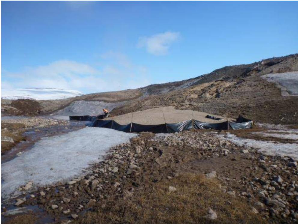
Photo 1 – May 29 th 2016. Silt fence installation around sediment deposit from slumping stream bank along Camp Lake Tributary #1.
