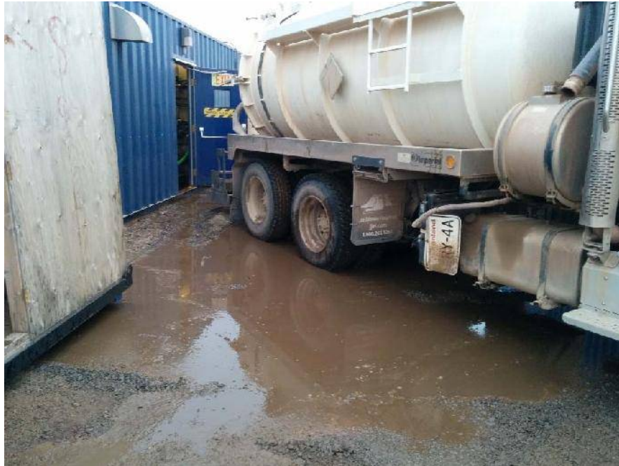
Photo 1. Spill contained to WWTP pad and vacuum truck used to suck up free liquid September 6 th 2016.
