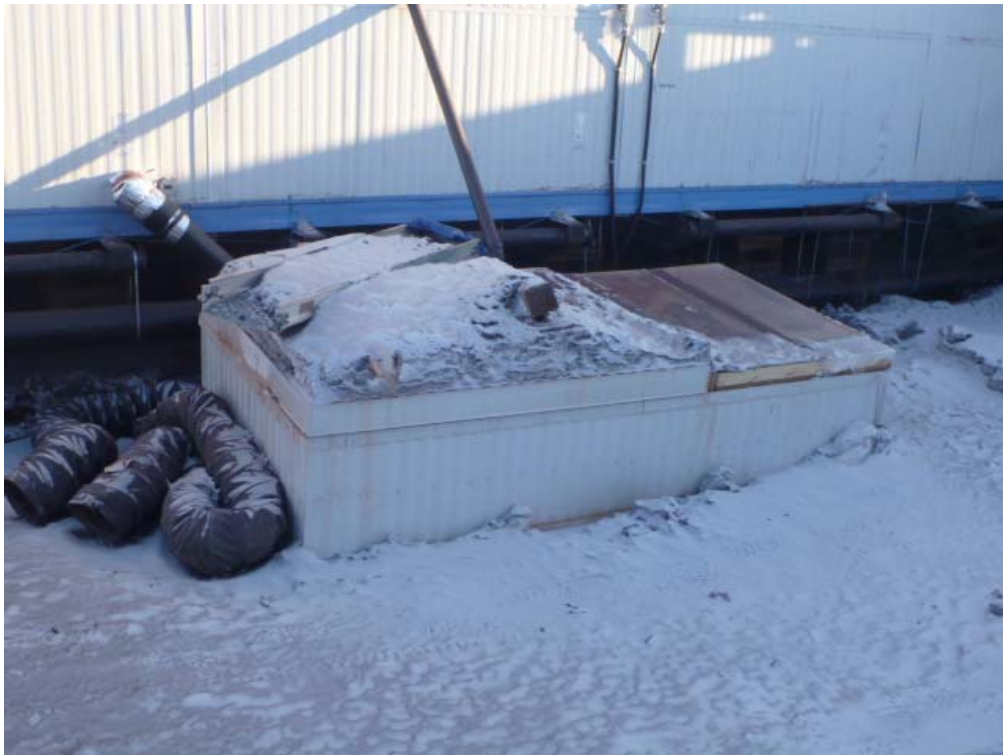
Photo 2 – Lift Station Spill Post Clean Up
