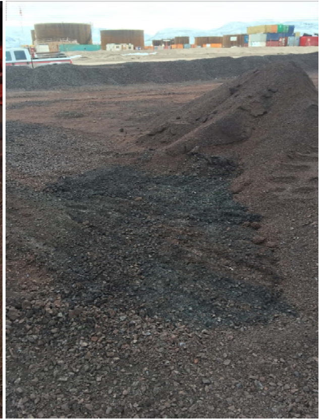
Photo 2– Spill Location after Cleanup
