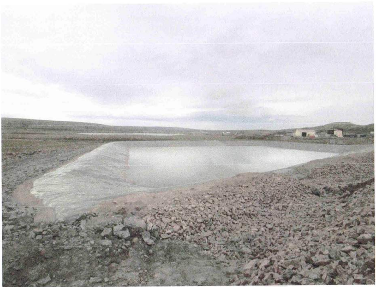
Crusher Pad Drainage Containment
