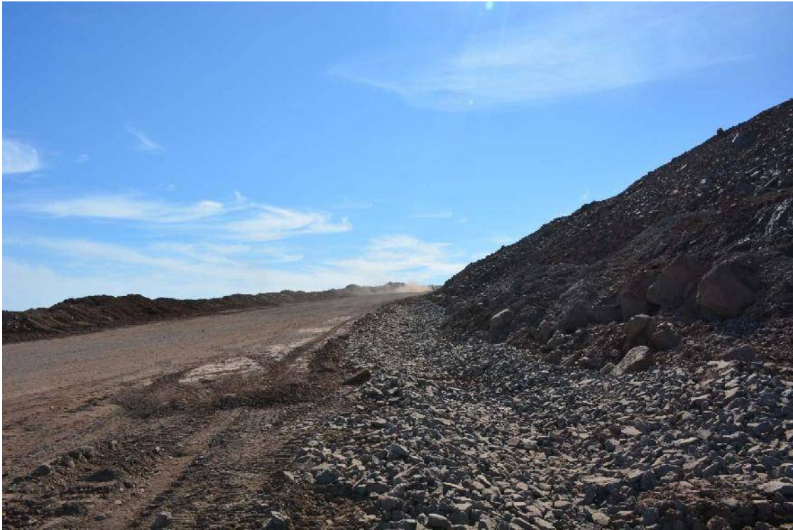
Photo 4 - New ditch with geotextile and rip rap up from Km 108.5. Picture taken on July 5, 2016
