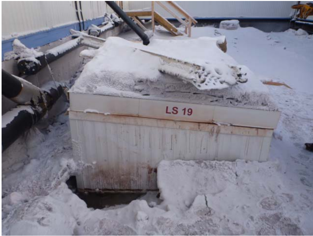
Photo 1 – Lift Station Spill
