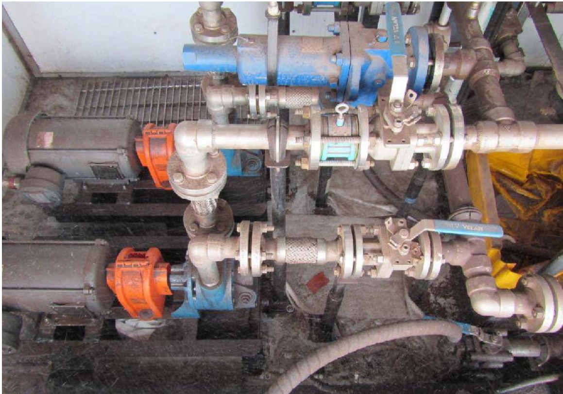
Photo 2 – Spill Contained within Module
