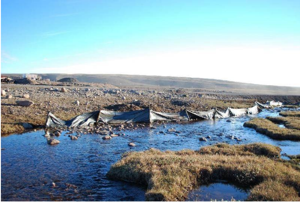
Photo 1 – Silt fence installation along road to prevent road runoff from directly discharging into Sheardown Lake Tributary (SDLT) near CV186.
