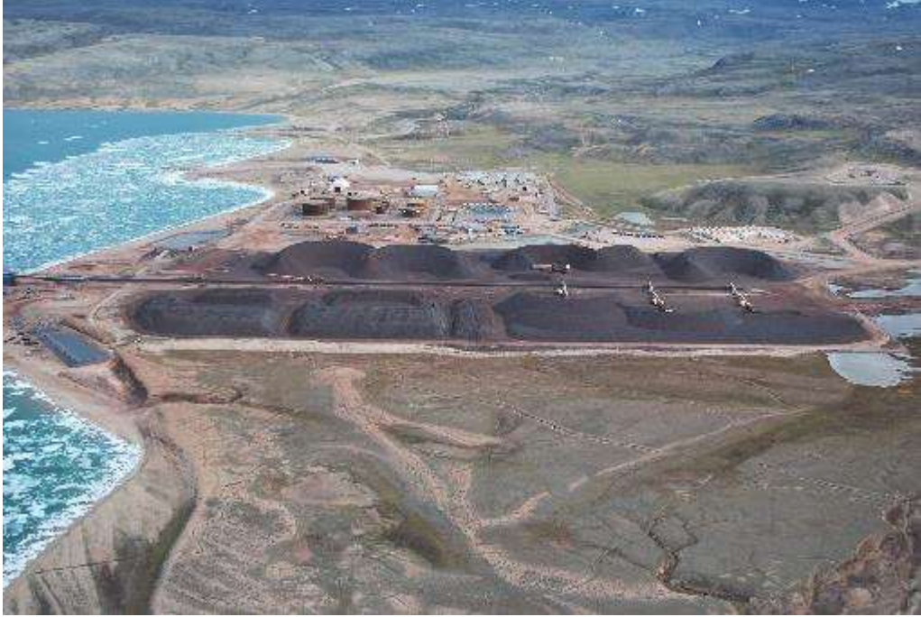
Photo 3 – Aerial view of completed ditch work at the Milne Port Ore Pad on July 18, 2016
