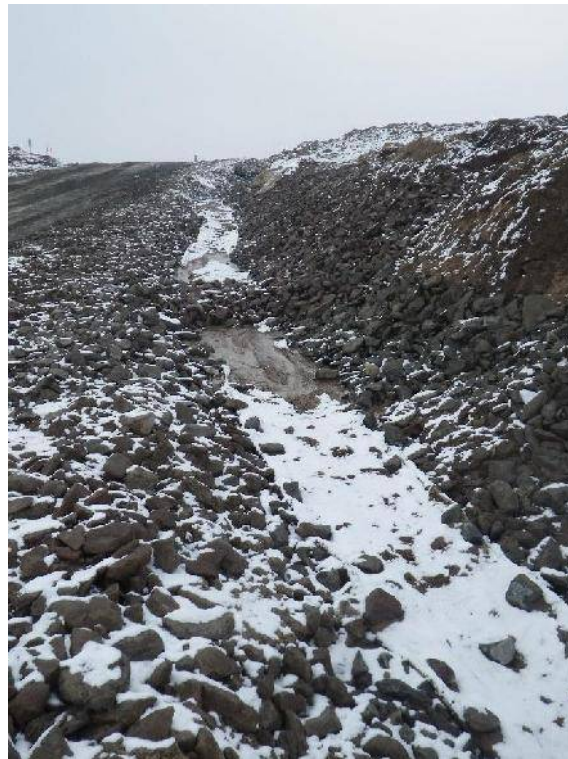
Photo 2 – Swale draining airstrip runoff lined with 6" aggregate and treated jute to capture sediments.
