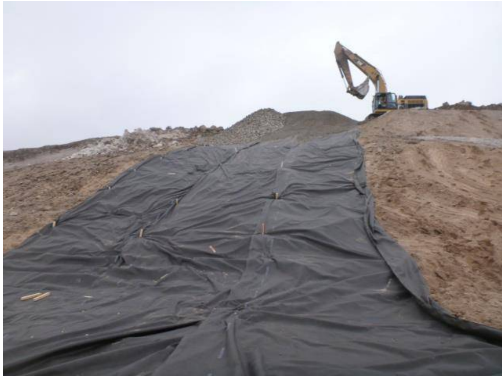
Photo 3 – June 3 rd 2016. Slumping stream bank lined with geotextile to protect underlying soil from erosion.
