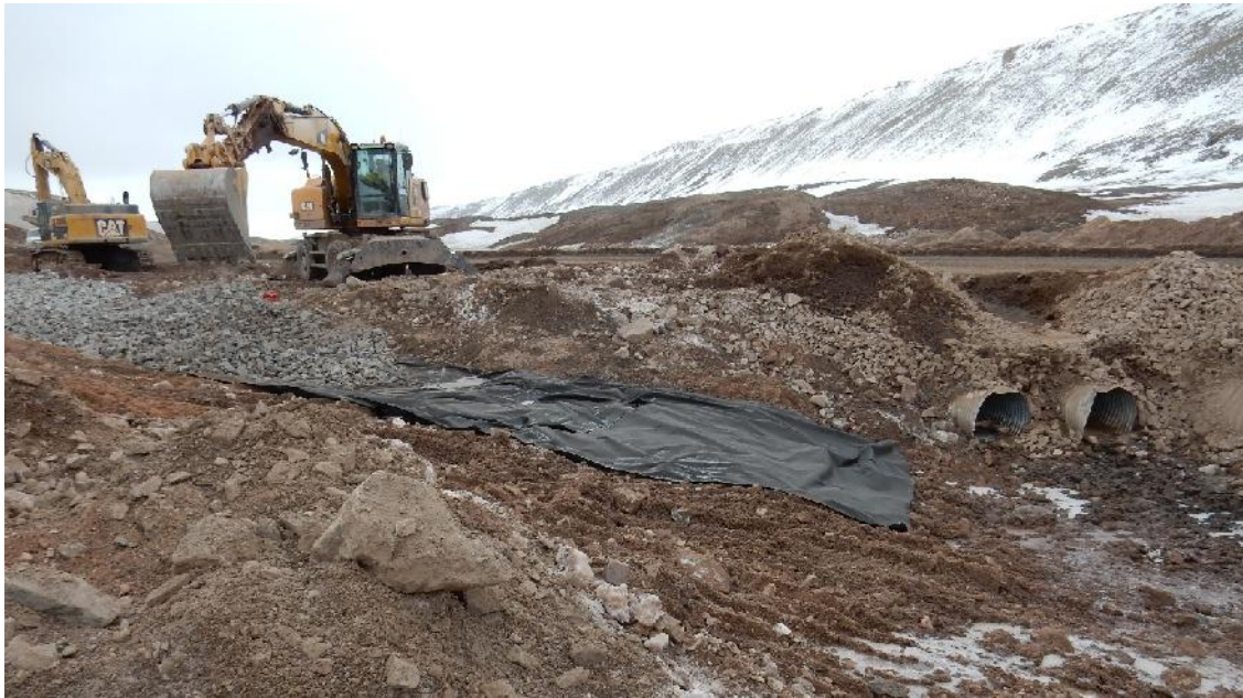
PHOTO 7 – Milne Port Tote Road Km 90 Ditch and Culvert Repair and Armoring, June 2016
