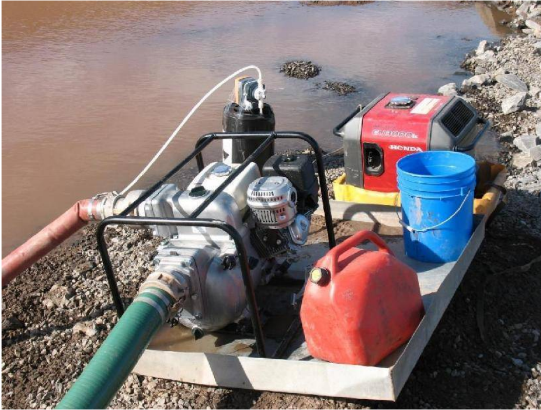
Photo 3 – Flocculant dosing system treating water upstream of Check Dam #4.
