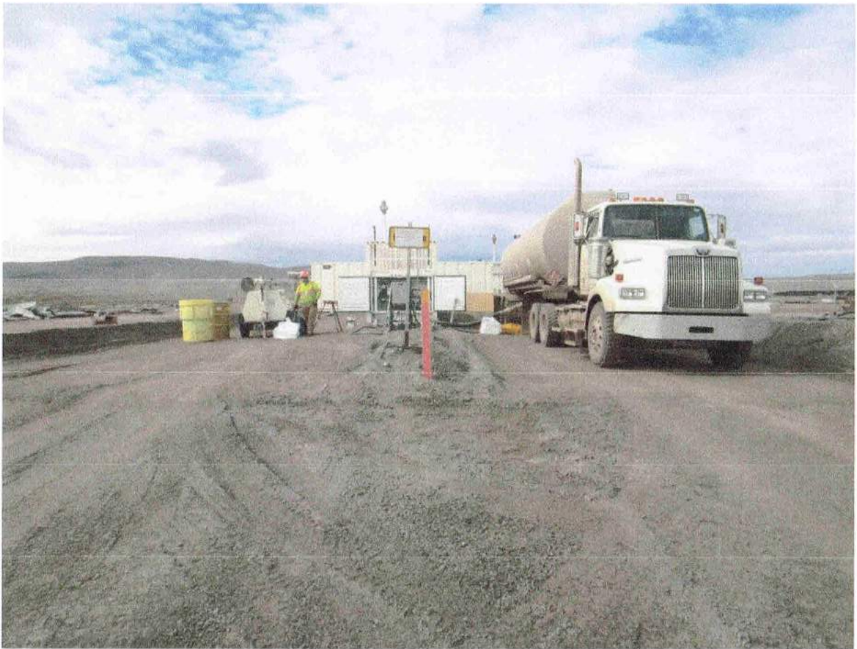
Fuelling Facility Containment
