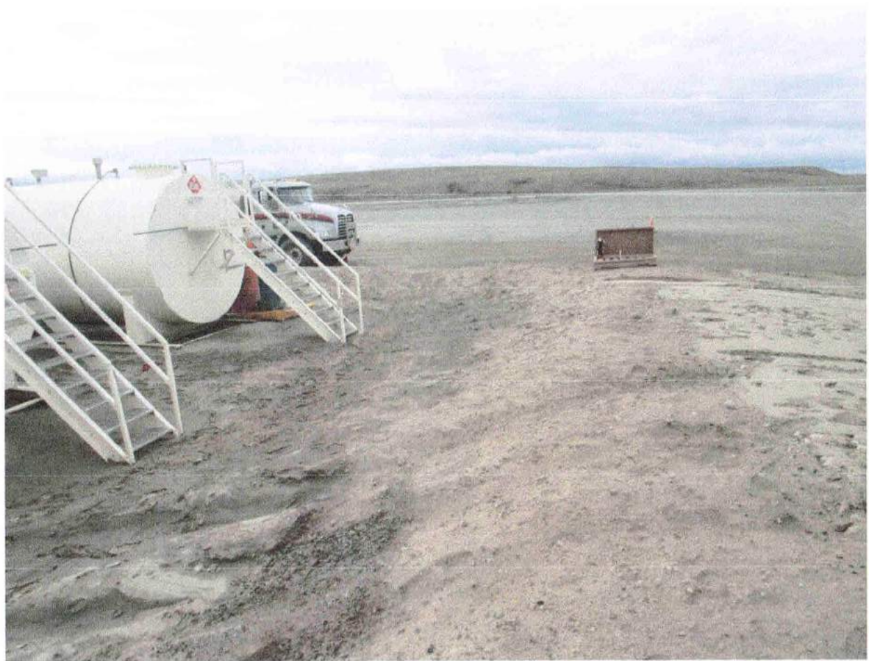
Jet "A" Fuel Containment
