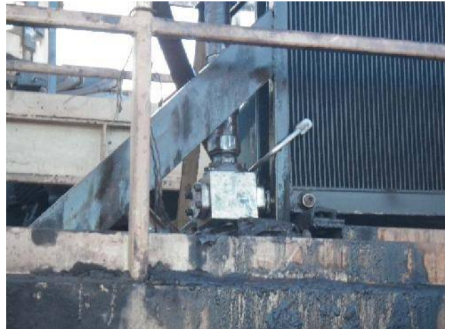
Photo 2 – Location of Hose Failure
