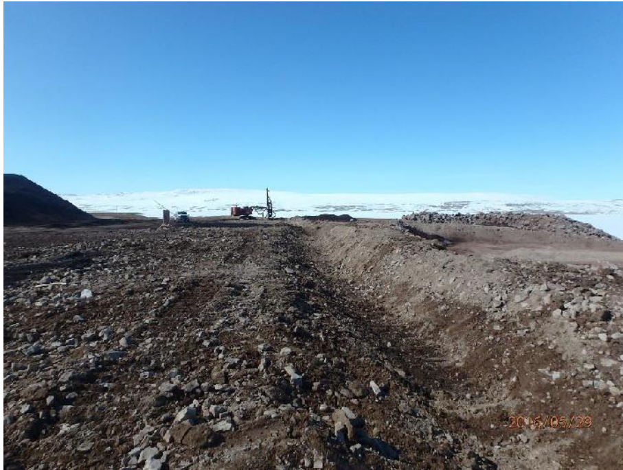
Figure 6: View looking North West with Swale, Berm and Drill Rig in Background
