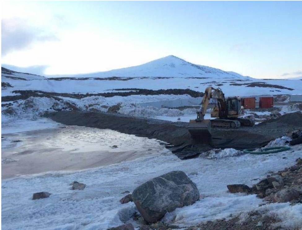
Photo 1– April 28 th 2016. Construction of Check Dam # 4 near the end of Magazine Access Road.
