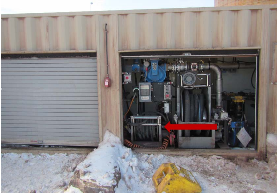
Photo 1 - Source of release – Secondary (back-up) fuel supply line
