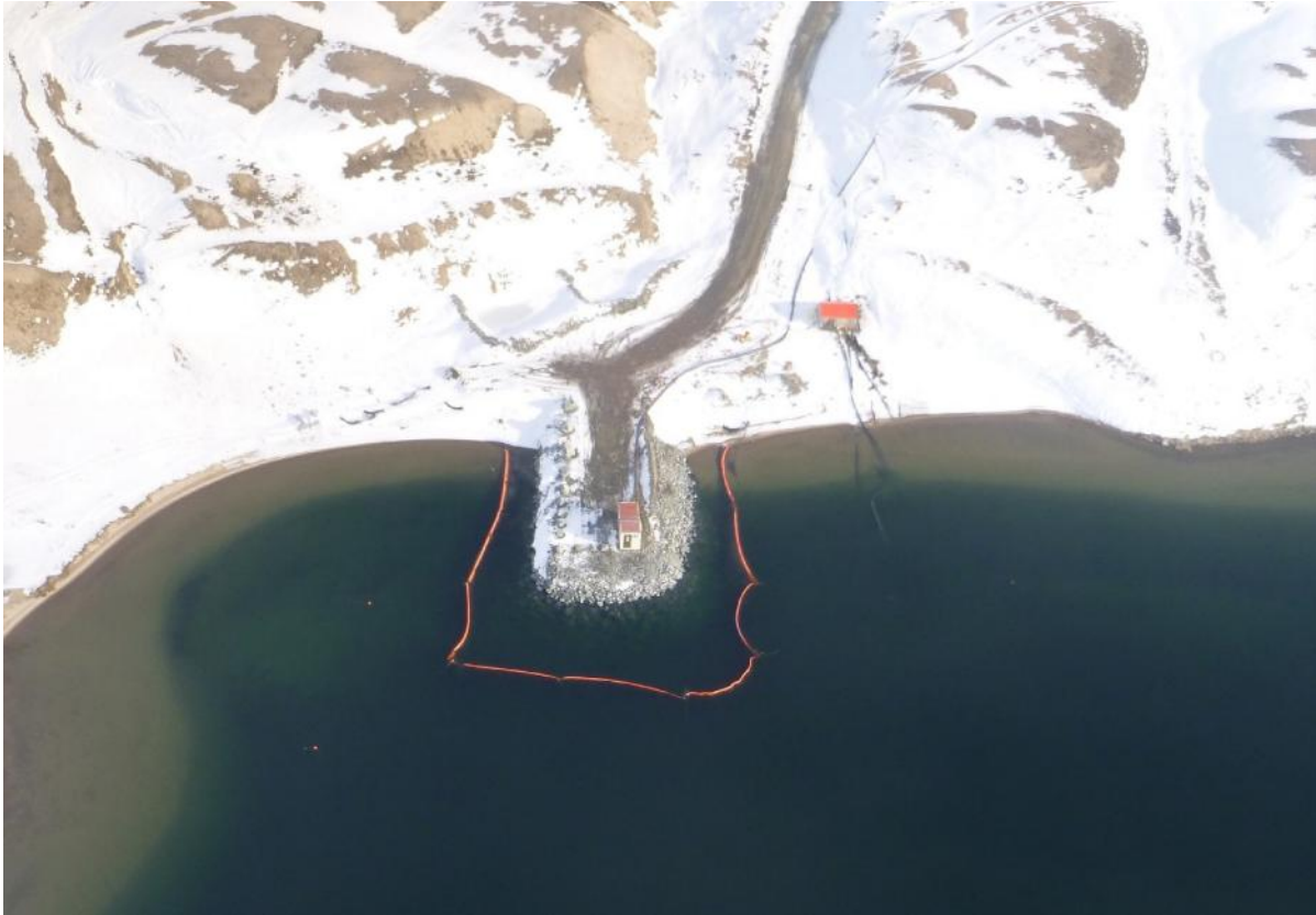
PHOTO 13 - Mary River Mine Site Jetty Repair Completed with Sedimentation Mitigation Measure in Place September 2016
