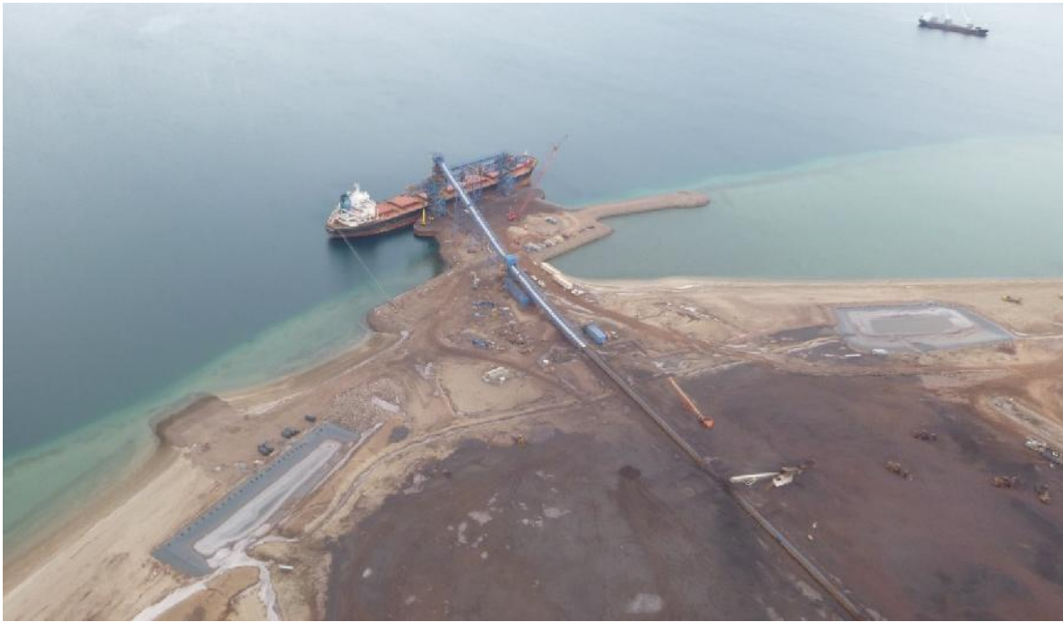
PHOTO 11 - Aerial view of the Milne Port Ship Loader and Sedimentation Ponds, September 2016
