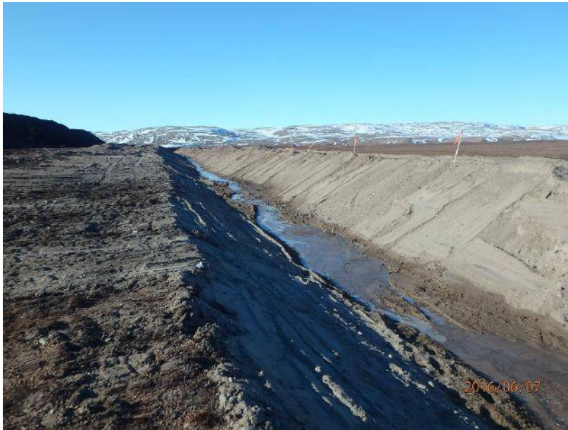
Figure 1: View looking South West showing Stockpile, Stockpile Pad, Drainage Ditch and Berm
