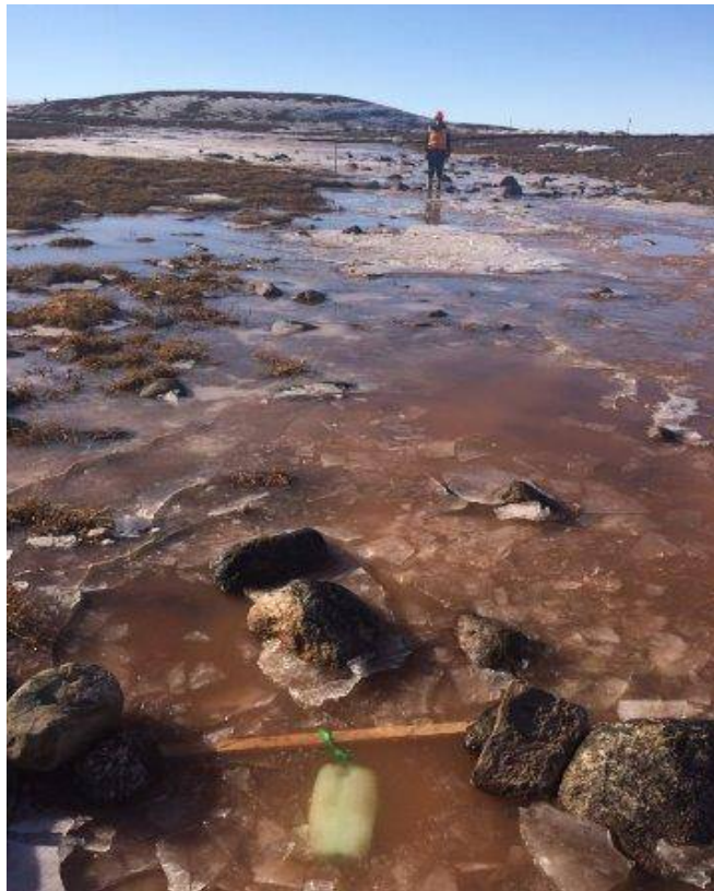
Photo 2 – May 9 th 2016. Flocculant stations installed along Sheardown Lake Tributary SDLT and LDFG.
