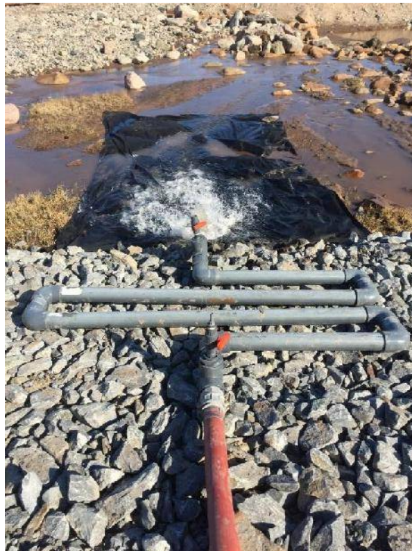
Photo 4 – Discharge of flocculant dosing system at Check Dam #4.
