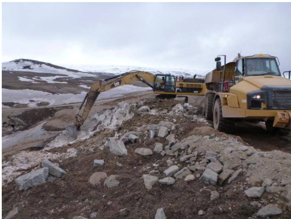
Photo 2 – June 3 rd 2016. Snow along slumping slope face and sediment deposit removed.
