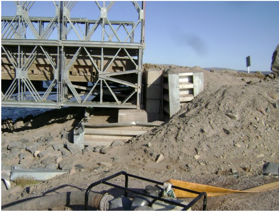
Photo 34 (2715): KM 80 Bridge, south abutment. Note tilting of upper bin wall.
