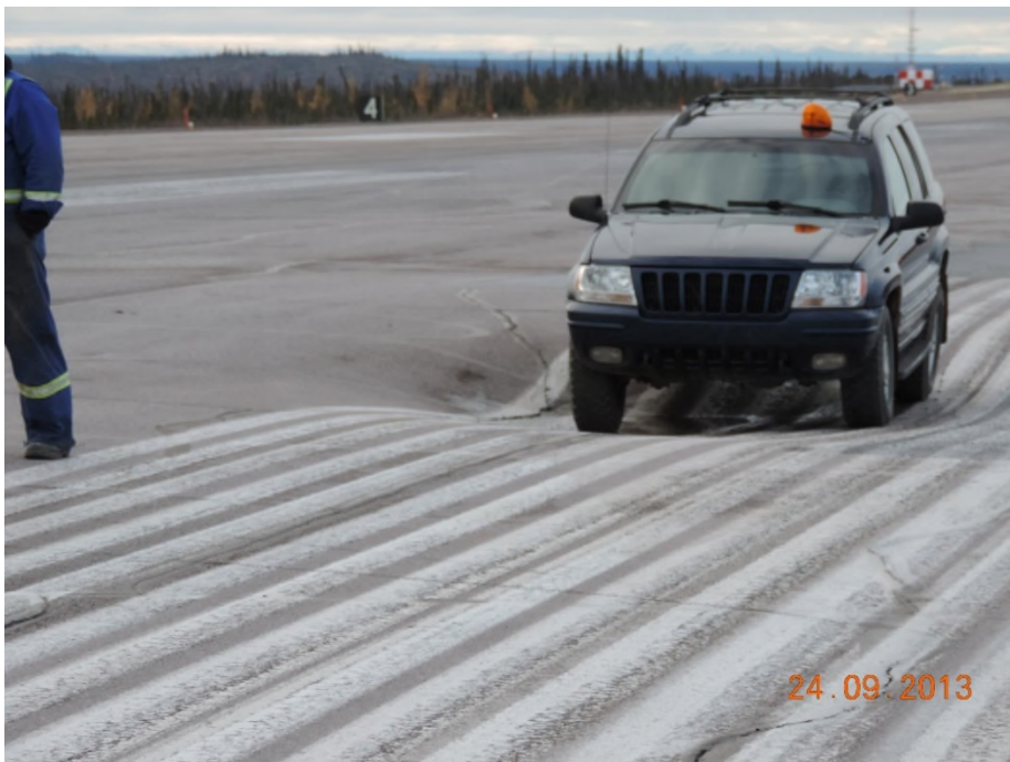
Photo 7: Extreme settlement of the runway at the Inuvik, NT airport. Settlement appeared overnight. Investigation revealed that the settlement occurred due to thaw of an ice wedge below the embankment. The embankment had bridged the void left by the thaw for a considerable length of time (likely several years).
