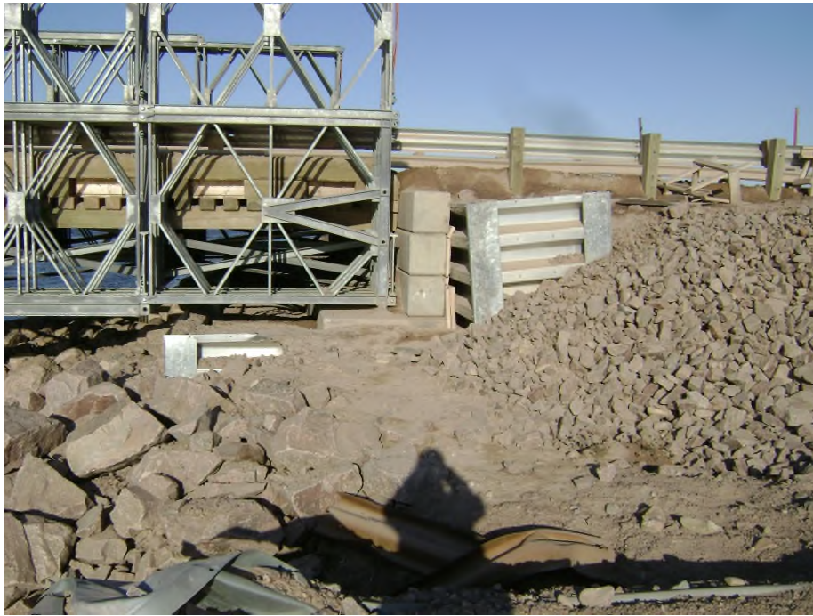
Photo 30 (2683): KM 17 Bridge, east abutment. Note tilting of upper bin wall.
