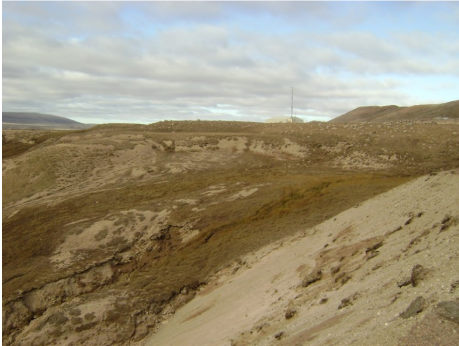
Photo 40 (2528): KM 4.0 erosion location immediately below the culvert on the north side of the terrace.
