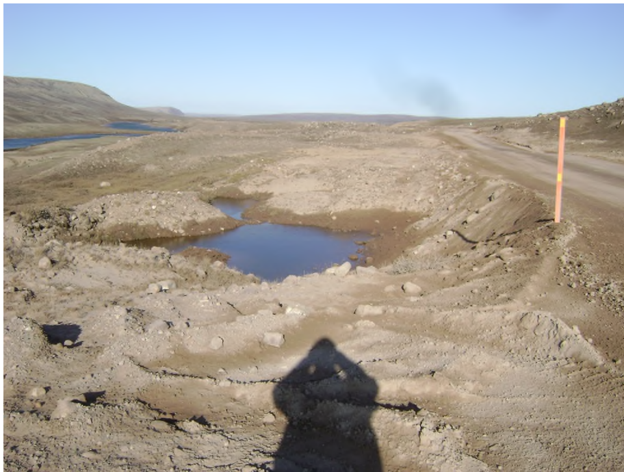
Photo 15 (2693): Pit at KM 21.9 (Figure 3), continued thaw of ice-rich material exacerbated by the ponding leading to steep side slope and instability of the embankment.
