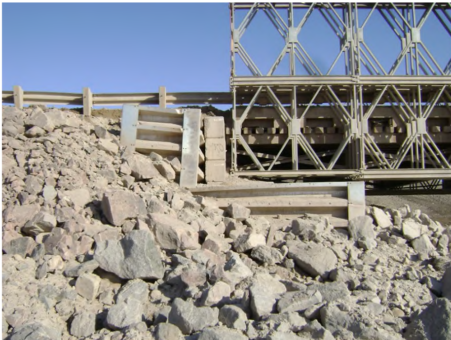
Photo 31 (2683): KM 63 Bridge, north abutment. Note tilting of upper bin wall.
