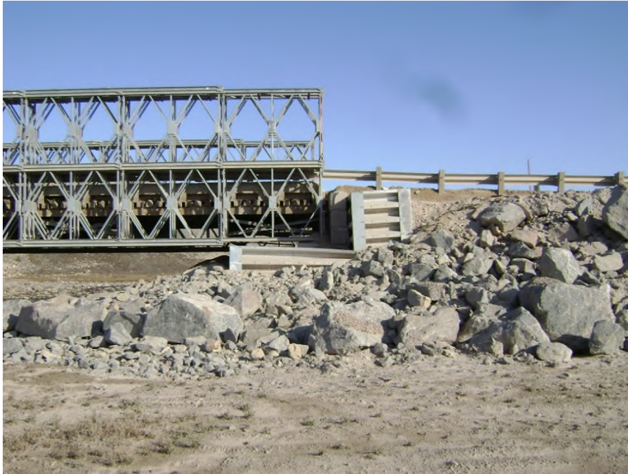
Photo 32 (2708): KM 64 Bridge, south abutment. Note tilting of upper bin wall.
