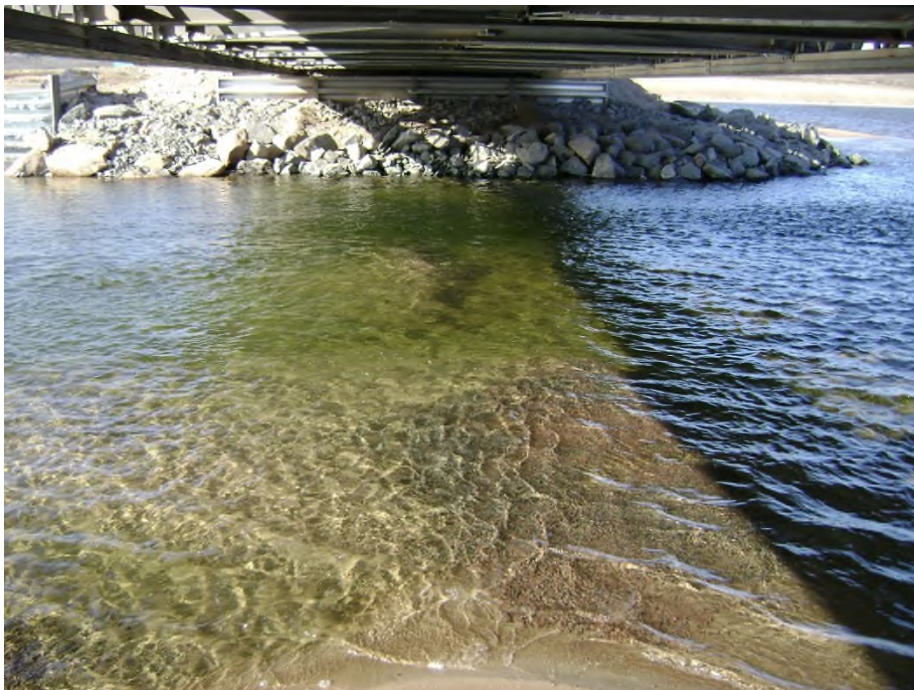
Photo 35 (2718): KM 80 Bridge, road surfacing gravel that has fallen through the centerline joint in the bridge deck and is visible in the river.
